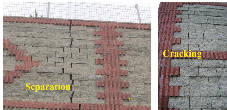
20 21 22 Figure 2 Types of block movement a) Separation, b) Cracking
