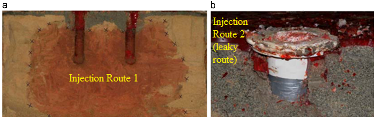
Fig. 16. (a) Grout penetration around injection wells and (b) leaked gel between the cover and the bentonite layer.
